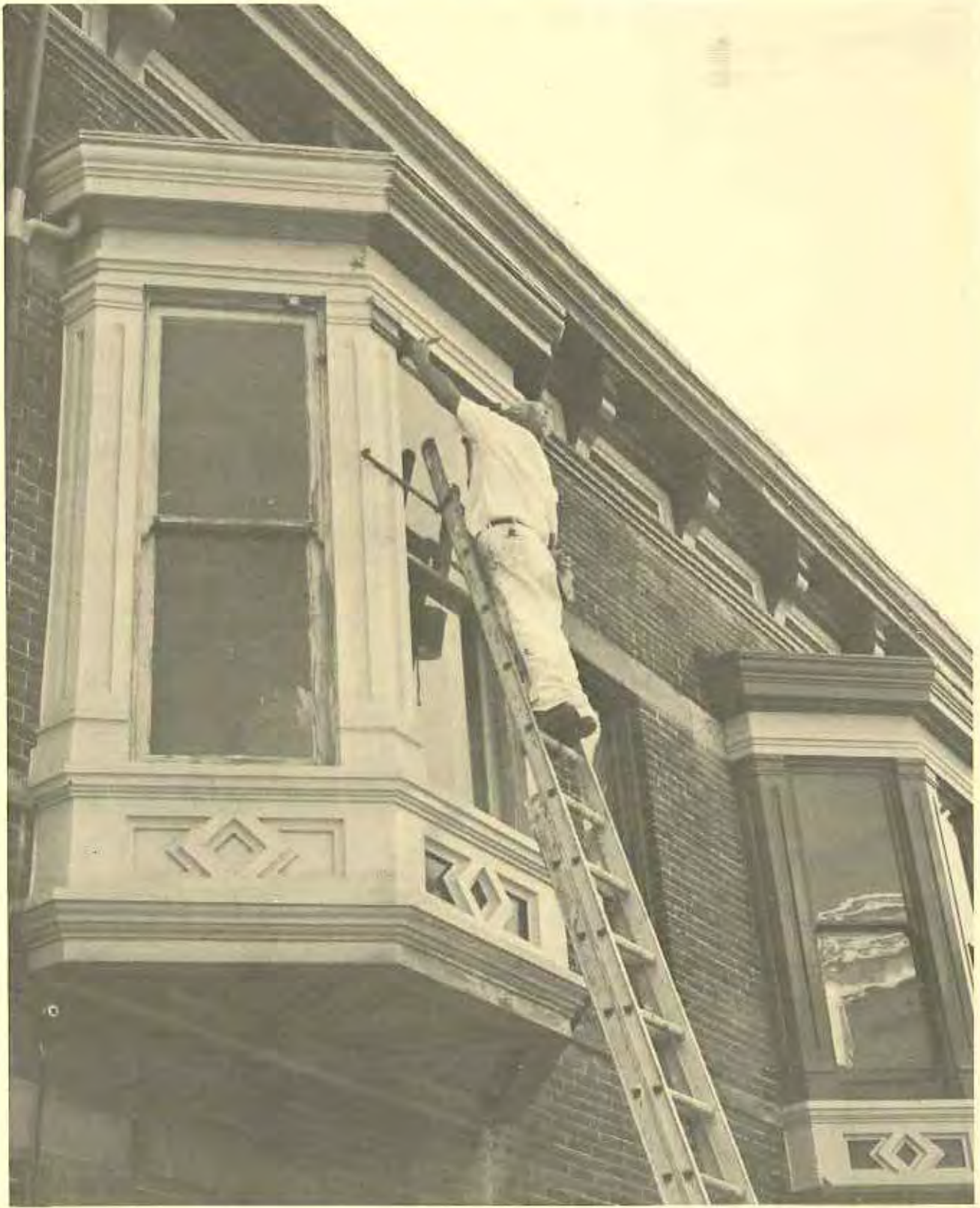
Restoration and maintenance in progress. The character of the street and the charm it exudes will be largely dependent on the success of preserving existing architectural quality worth saving and adding the necessary contemporary infill.
