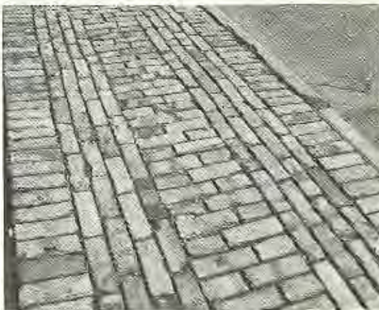
Caution is advised in brickwork of this type because of its irregular surface.
