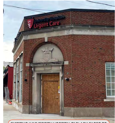
EXISTING "UNIVERSITY HOSPITALS" BLACK FACES TO BE REMOVED AND REPLACED WITH NEW
